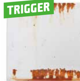
Impressive rust protection. Bottom edge, where it was wiped proved most vulnerable.
